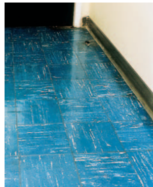
Asbestos-containing floor tiles
