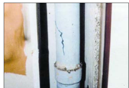
Sometimes, the joints are sealed with asbestos string.
